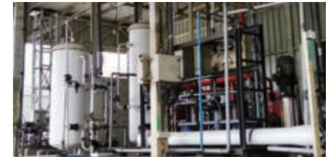
DMF water treatment tank and RO treatment facility
